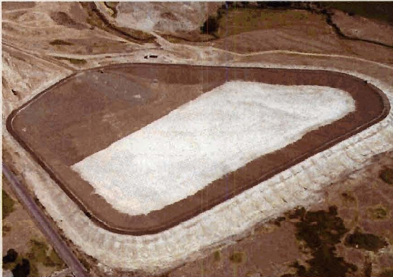
The 59.29 re-regulation reservoir is nearly complete. The reservoir will start filling in very early July with full operation expected by late July.
