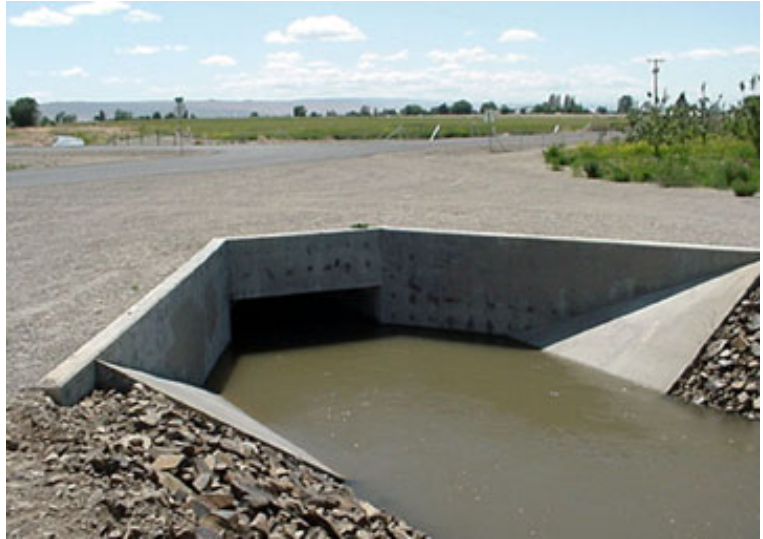
This picture shows the new box culvert installed on the Mabton Lateral. The new culvert allows for a wider crossing, improving safety for motorists. The project is being hailed as a successful example of how different entities can work together to improve mutually beneficial facilities.
