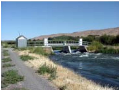
Mile 2.92 was retrofitted with automated gates which allow for adjustments through wireless access.
